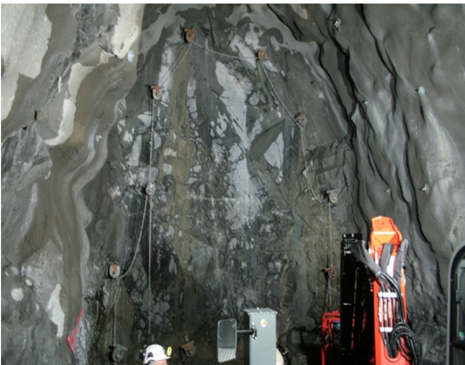
Stand pipes mounted in face
