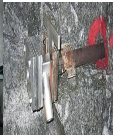
Water diverter mounted on stand pipe
